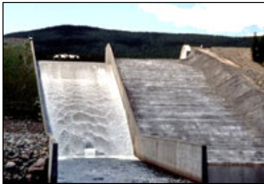
Figure 10: Typical Reinforced Concrete Service Chute and Auxiliary RCC Emergency Overflow Chute (Courtesy of www.cement.org/basics/concreteproducts-rcc.asp )
