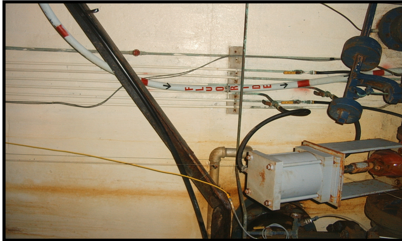
Fluoride Injection at Clearwell
