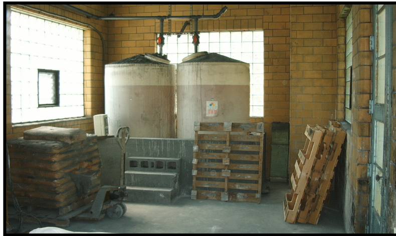
Bulk Coagulant Tanks
