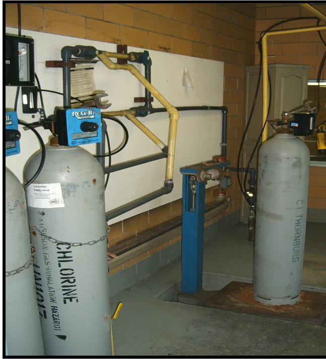
Chlorine Gas Feed System
