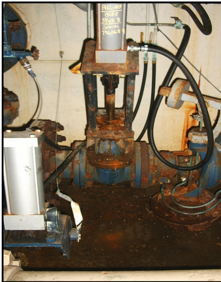
Filter Control Valve
