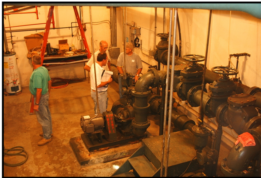
Raw Water Pumps and Piping
