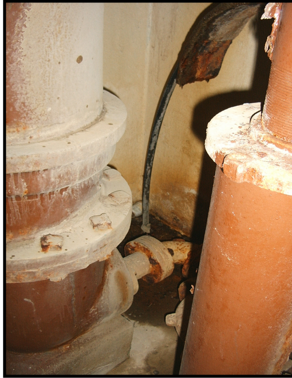
Chlorine Injection Point at Clearwell
