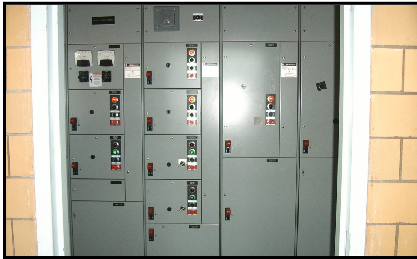
Electric Service Distribution
