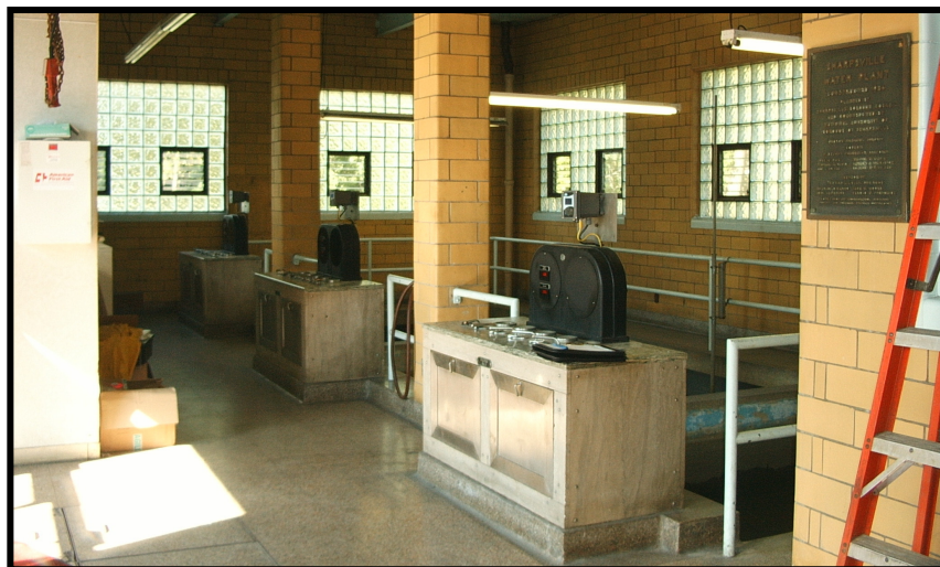
Filters on Operating Floor
