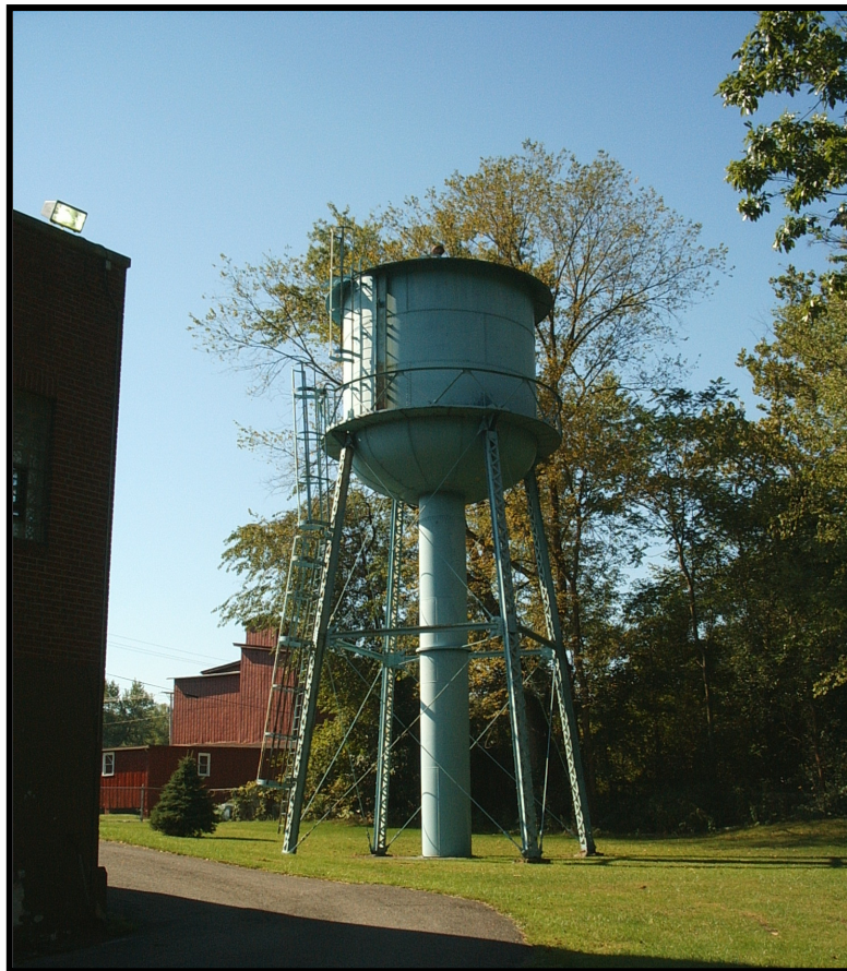
Backwash Storage Tank
