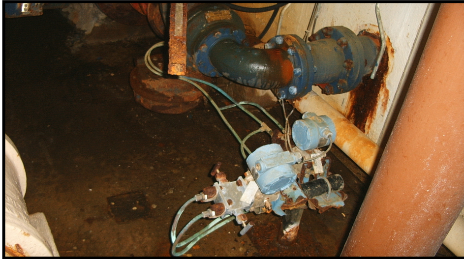
Filter Flow Meter
