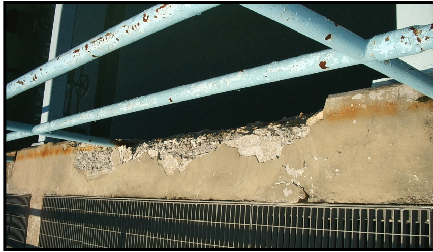
Deterioration of Sedimentation Basin Concrete
